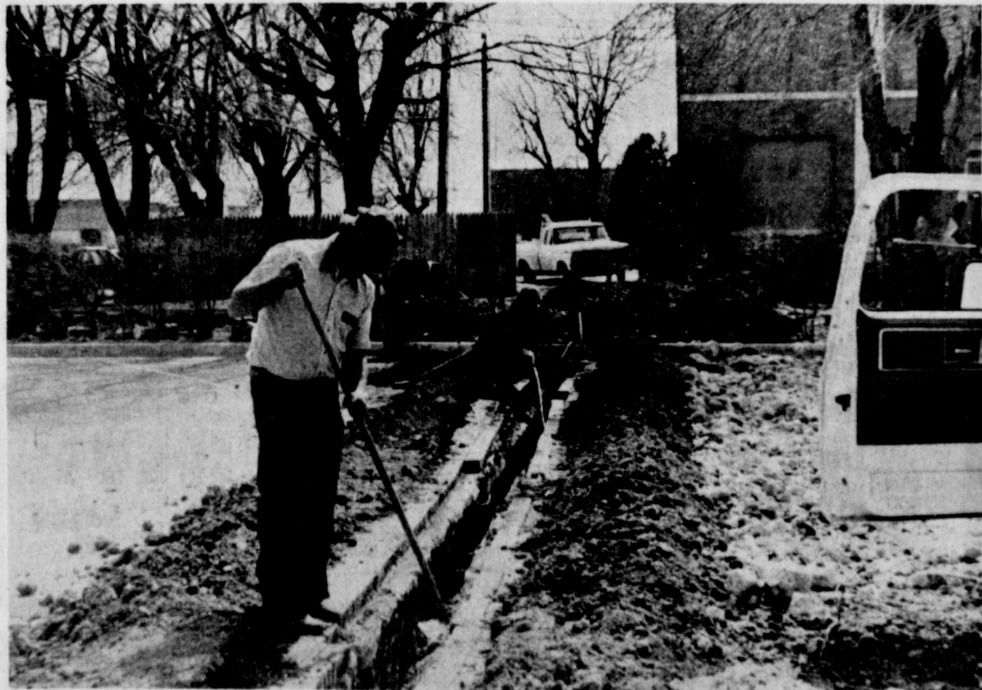
MISSOURI STREET, adjacent to the courthouse square, was blocked Friday by contractors installing a new water
