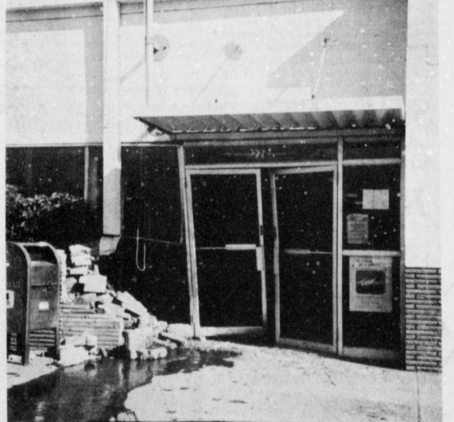
DRIVE-IN WINDOW — The Floydada Post Office takes on a new appearance after a motorist accidentally drove through the front doors Thursday.
