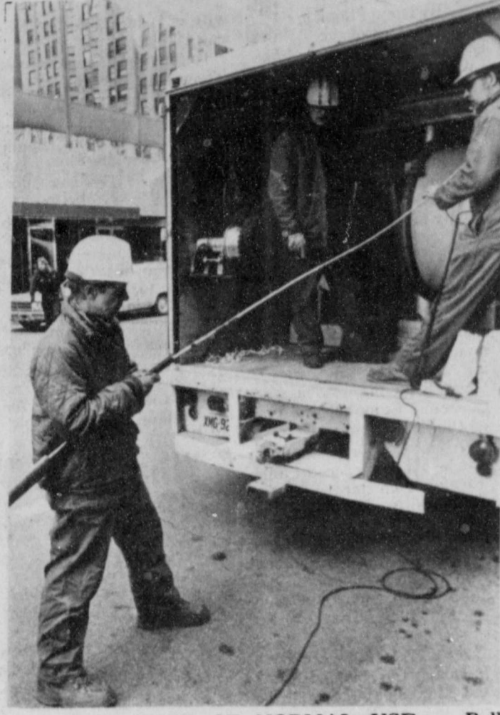
AFTER A YEAR OF NORMAL USE, a Bell Laboratories experiment in lightwave communications has exceeded expectations, with no "downtime" and virtually no transmission errors. The cable, which was installed in downtown Chicago, contains 24 glass fiber lightguides and is carrying voice, data and video signals on pulses of light.
