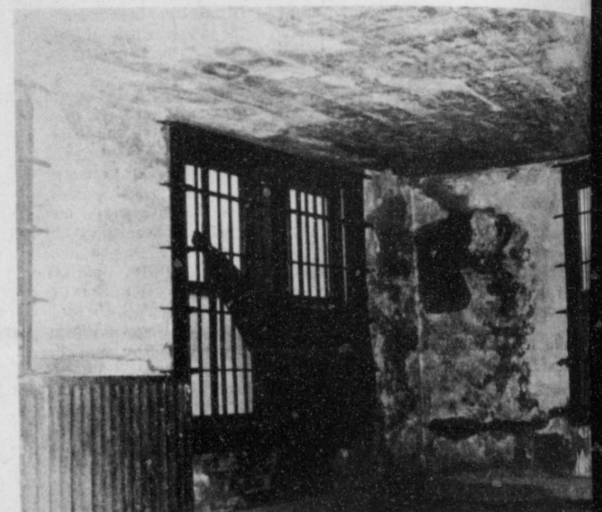
N.E. CORNER OF 3rd FLOOR cell block, missing plaster & mortar & ceiling due to rain seeping in through cracks in exterior walls & moisture from open showers located on the same floor.
