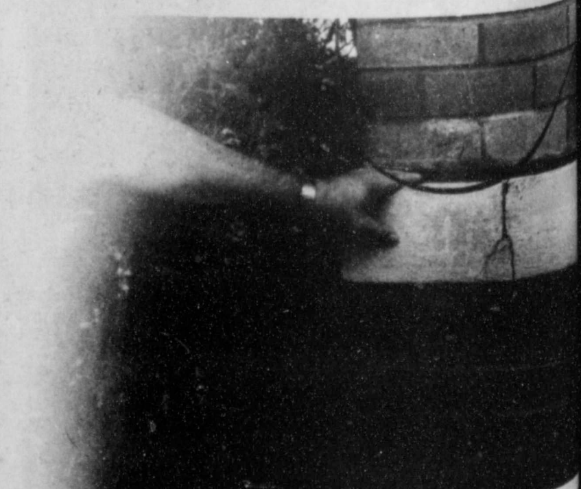
DEPUTY SHERIFF SHOWS large crack in n.w. corner of jail. Due to foundation settling.
