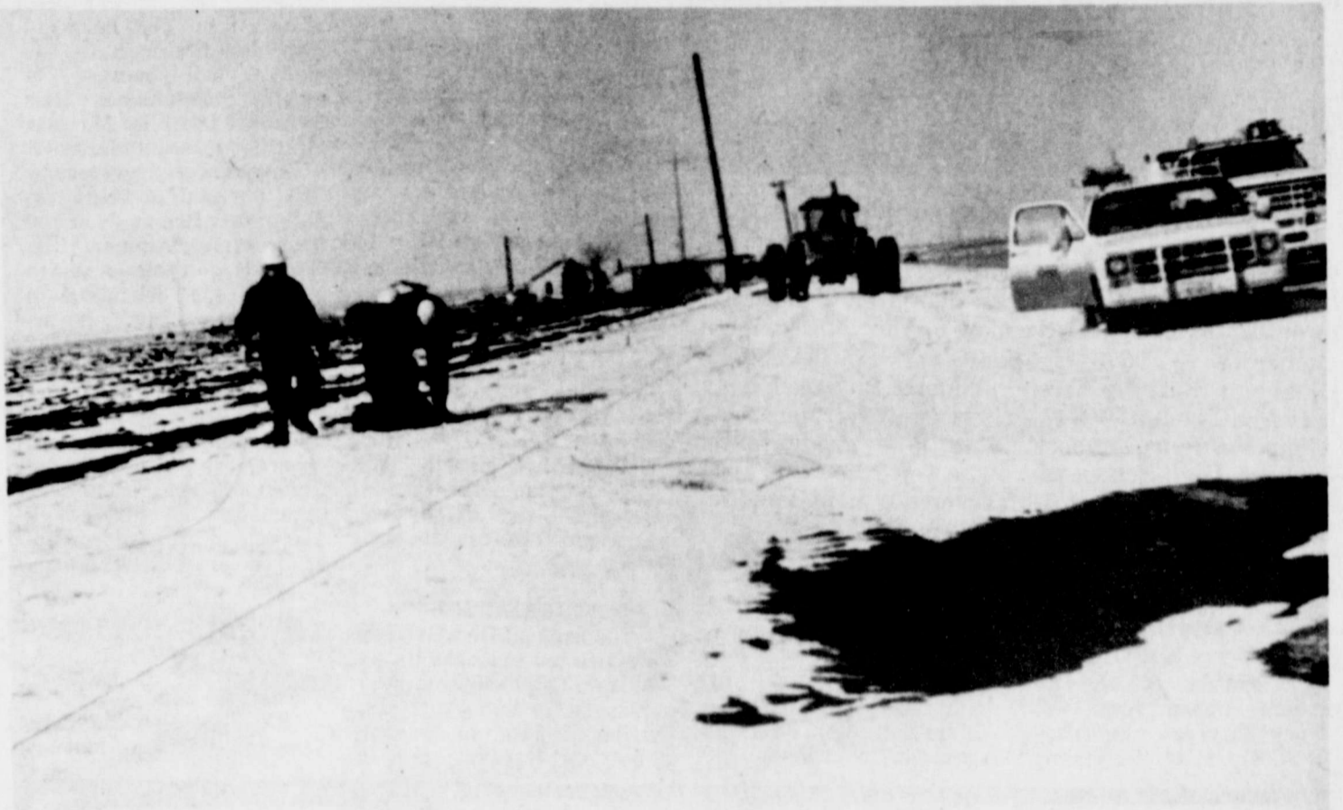
LIGHTHOUSE ELECTRIC linemen are pictured in the Silverton area rebuilding electric lines following costly ice damage. (Photo by Anthony Whitfill)
