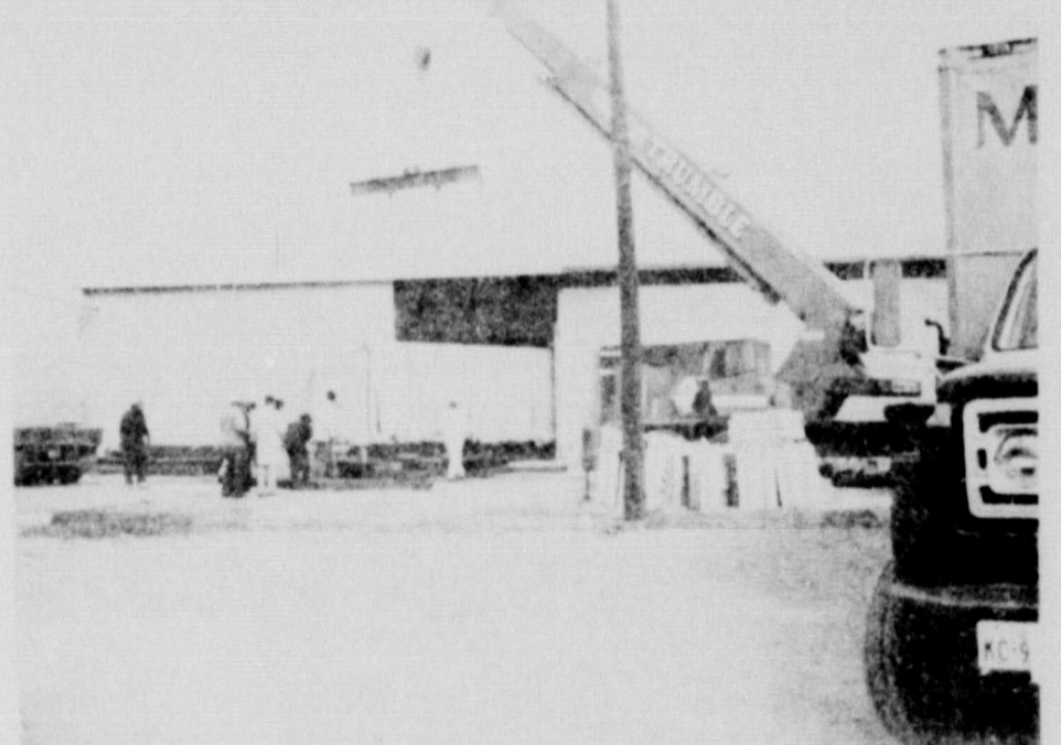
NEW "0 PLUS" equipment was unloaded and installed at the Bell Telephone plant in Floydada Friday morning. The new dialing system will soon be in service for this community. (Staff Photo)
