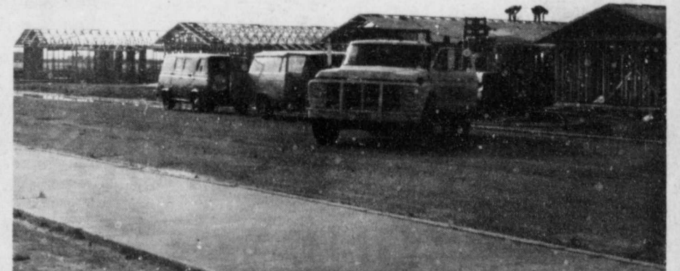
SIXTEEN NEW APARTMENTS are beginning to take shape just south of Duncan Elementary in Floydada. (Staff Photo).
