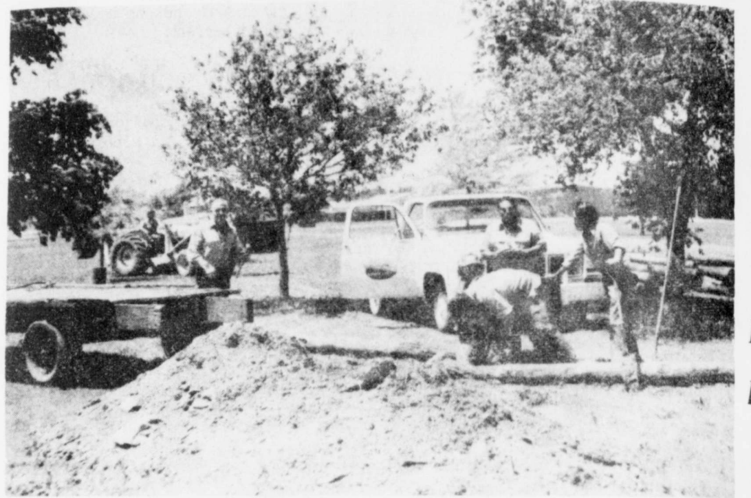
CITY OF FLOYDADA employees are pictured working on playground equipment for park east of the high school. A government grant is supplying part of the money for materials. (Staff Photo).
