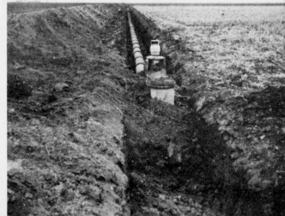
UNDER NEW REGULATIONS UP TO $7500 of irrigation practices such as the above irrigation pipeline may be cost-shared when other needed conservation practices are applied under the Great Plains Conservation Program.
