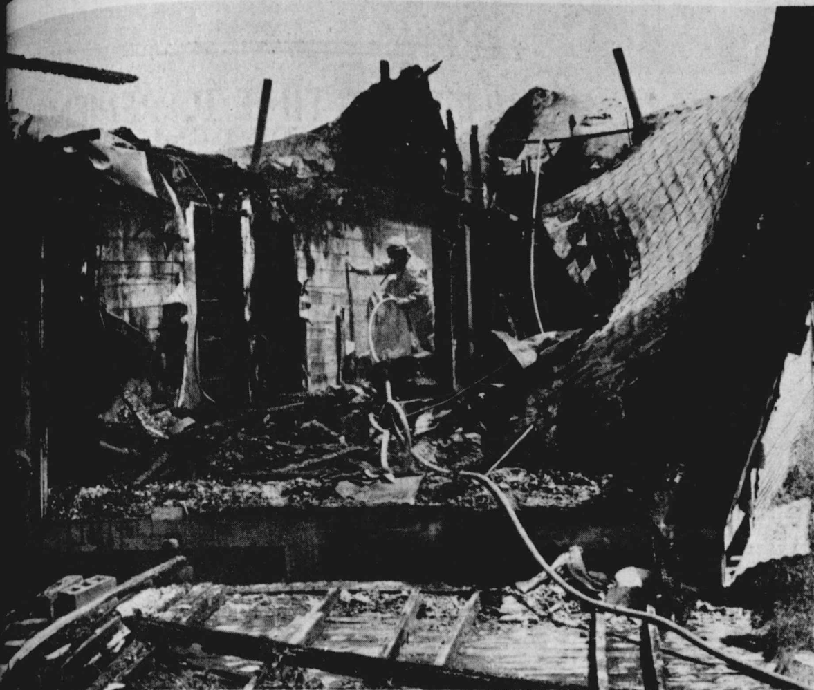
JONES RESIDENCE was heavily damaged by a fire that started early Monday morning and burned again that afternoon. (Staff Photo)
