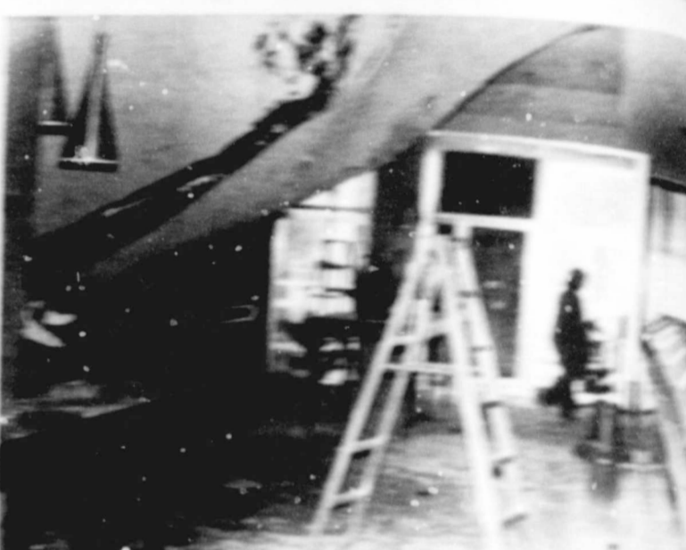
"THEY'RE FRANK BARROW'S DEN" under the Floydada First National Bank Saturday morning. Other photos showing extensive damage caused to the building.
