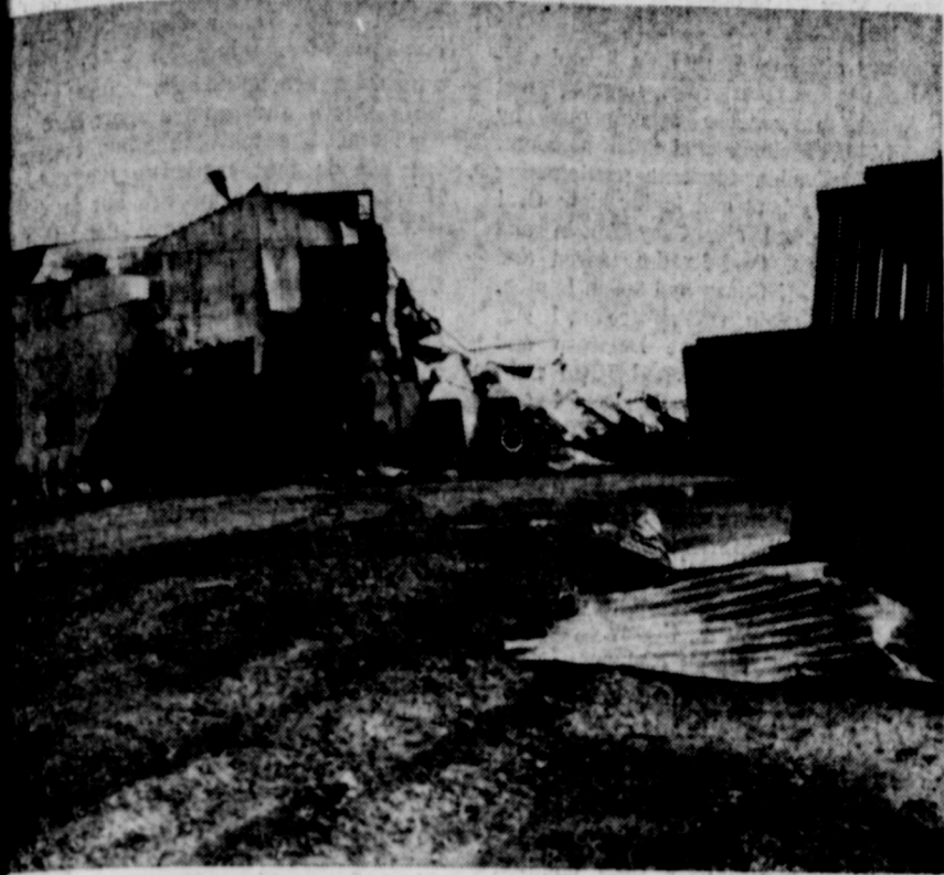
THIS COTTON GIN received major damage which put it beyond economical repair.
