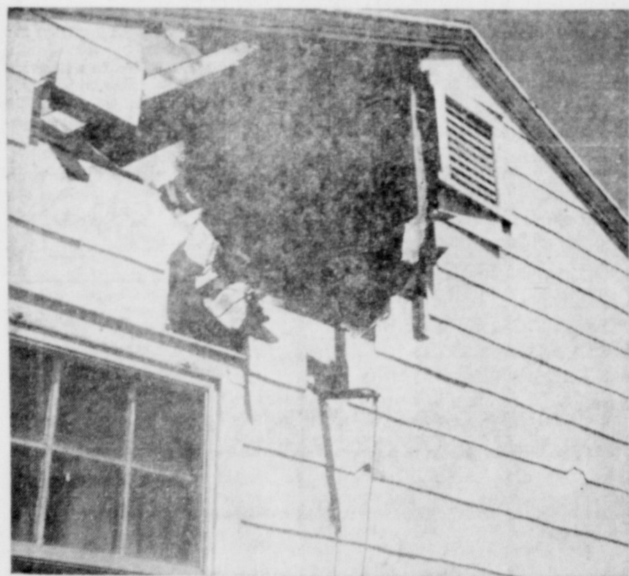
TORNADIC WINDS carried this sashweight from a school building to where it is stuck here. Cinder blocks from the same building made the gaping hole above it.
