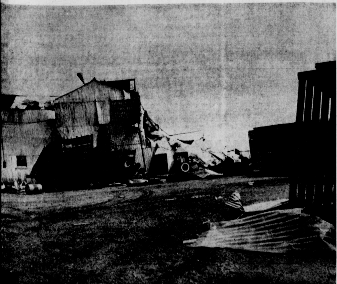
COTTON GINS and related equipment all received major damage.
