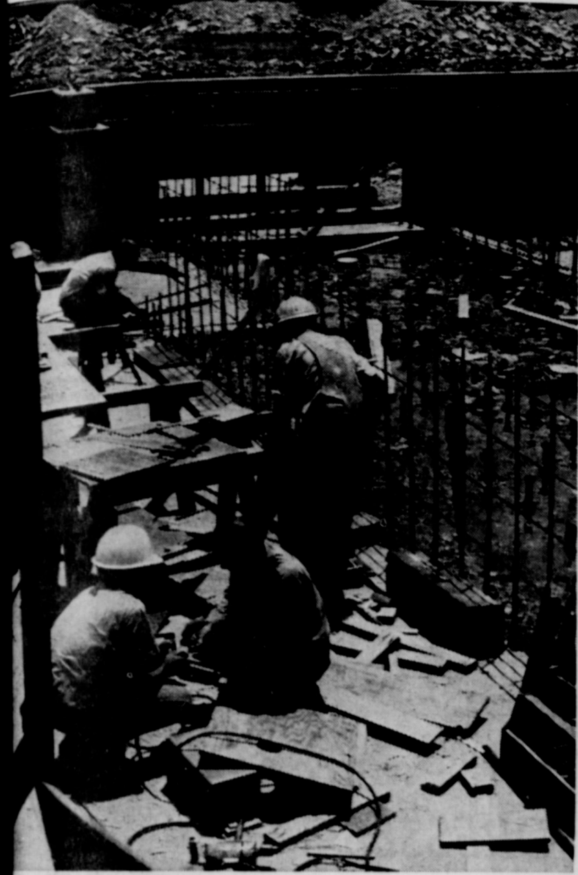
Work continues . . . WORK GOES AT a steady rate at the gas compressing station near Goodland. It is expected to be completed in September.
