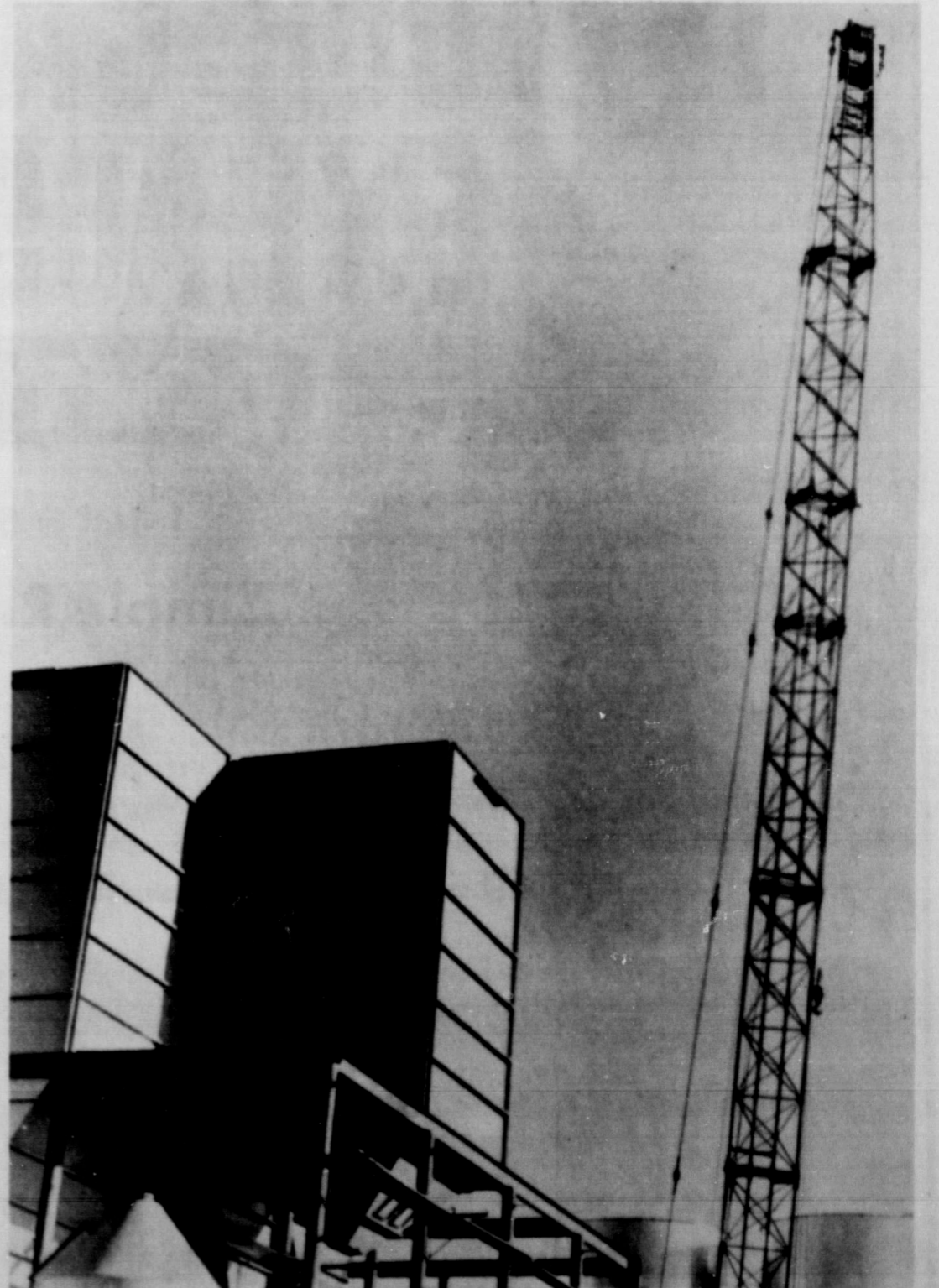
MILL GOING UP. . . A giant crane has been visible on the eastern edge of Friona lately, where the HI-Pro Feed Mill is being constructed. Much of the company's equipment has been on the premises, and the arduous task of assembling the mill has now begun.
