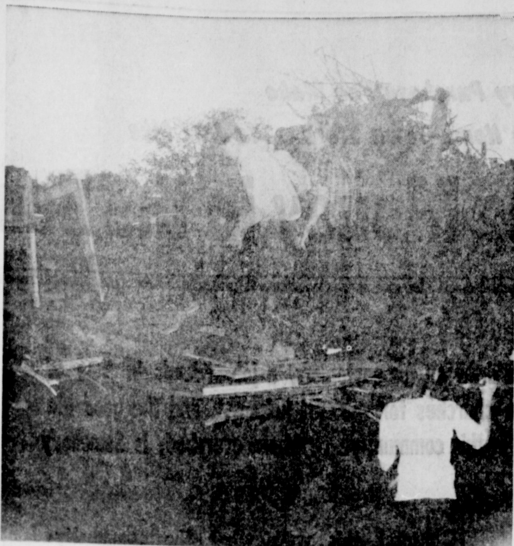
Lots of wood and work PILES OF WOOD and much physical labor went into the construction of the huge Homecoming bonfire Thursday night. The students from Morton High School vied class against class as to who could gather the most wood. The Sophomores won the $5 prize for the most wood, but put much work in the fire. TRIBUNE Photo
