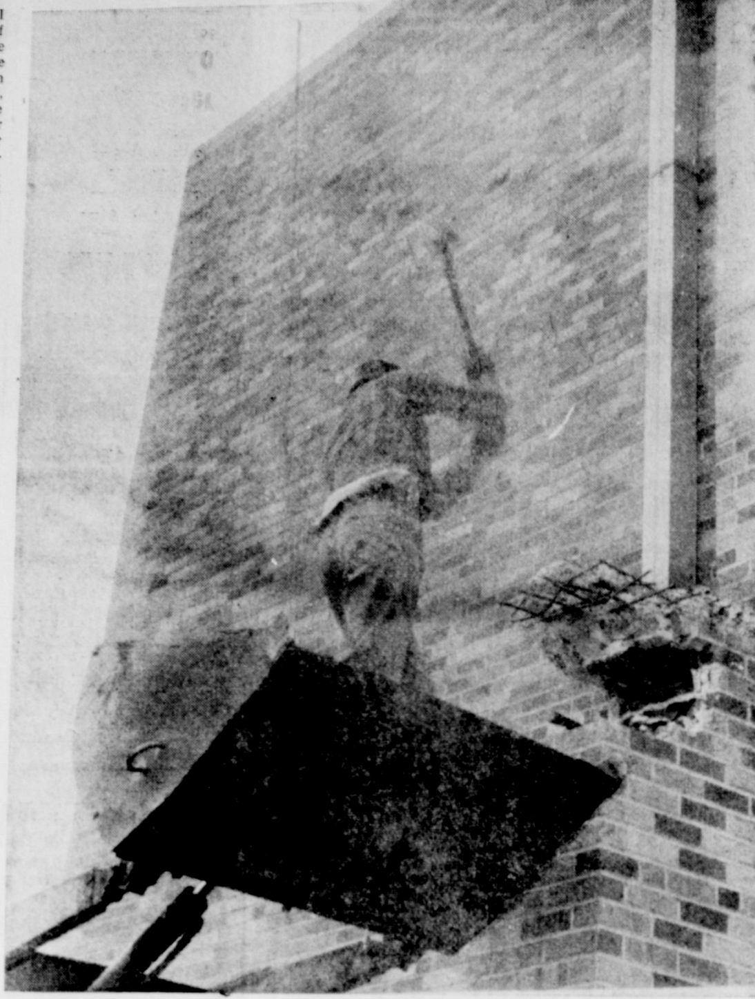
Work on addition the building will be extended and remodeled to accommodate more facilities. TRIBUNE Photo
