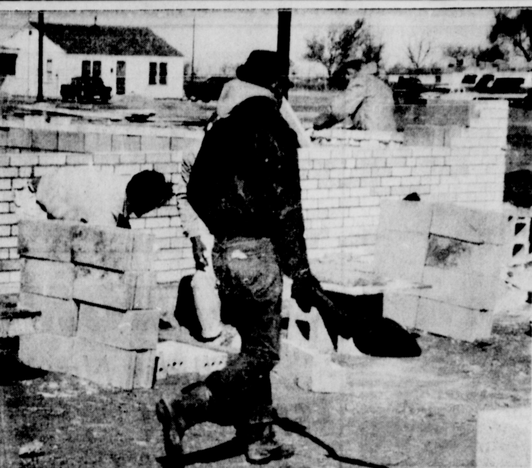
Building a school CONSTRUCTION WORKERS, aided by recent warm spring temperatures, are making rapid progress on the new Morton High School. The $400,000 job is expected to be ready for use at the beginning of the 1964-1965 school term. TRIBUNE Photo
