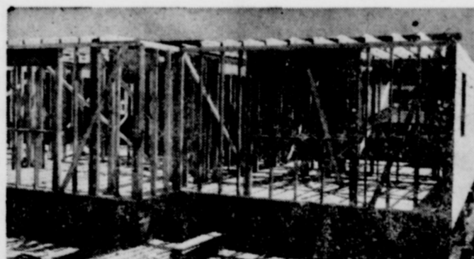
A quality house starts with a good floor. Note 2-inch sub-flooring and rigid corners at very beginning of this skillfully-built Avinger house.
