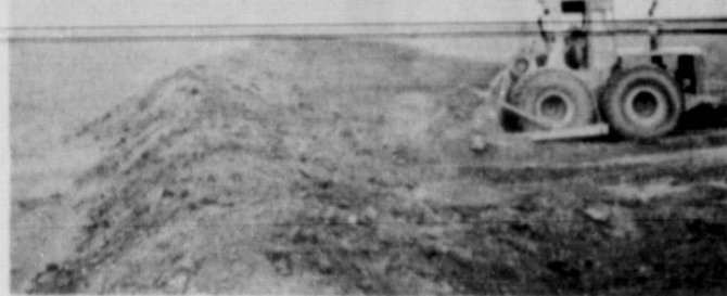
PARALLEL TERRACES, . . . M.C. Osborn has recently completed construction of parallel terraces as part of his conservation plan.
