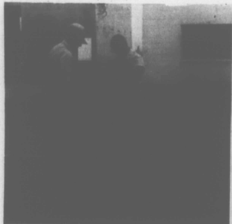
PICTURED ABOVE IS City Water Commissioner, Pete Phillips and John Hendrix repairing the six inch water main that broke on the west side of town. The water line goes down where Hi-way 84 is now about ten feet from the curb on the south side.
