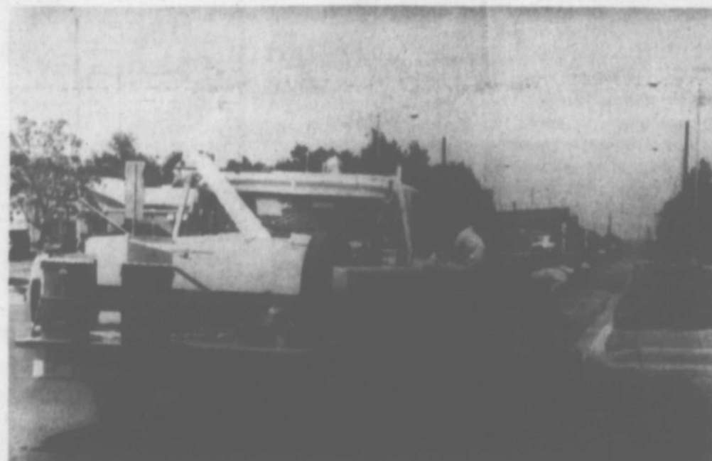
PARALLEL PARKING is now in effect on Main Street from First Avenue to Fifth Avenue on the east side; and angle parking on the west side from Hwy. 84 through Fourth Avenue. Painting corners yellow is Henry Scott. The yellow indicates no parking in that area. (Staff Photo)
