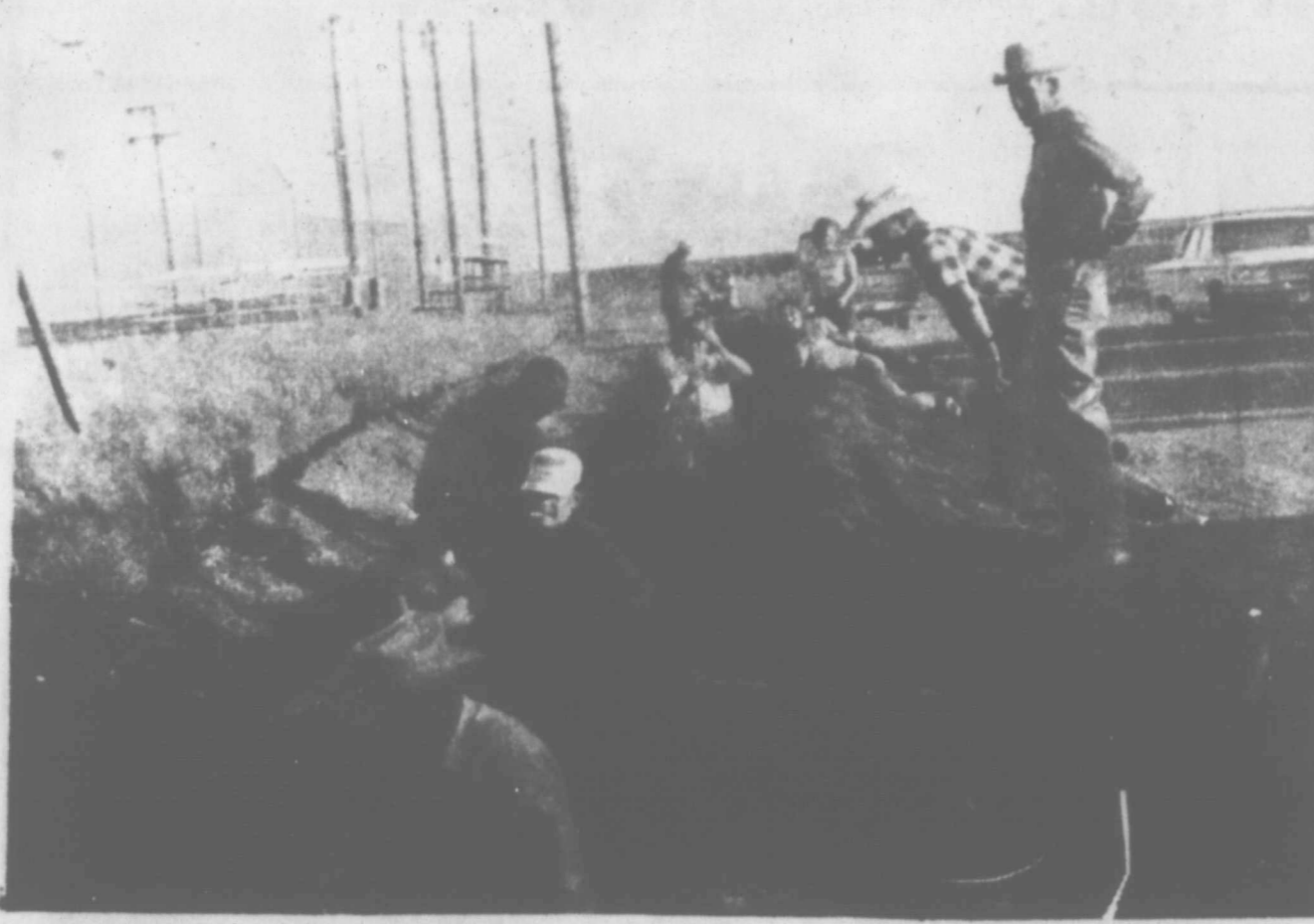
MODERN DITCH-DIGGER - Luna Snow is shown above operating the ditch digging machine at the Sudan Baseball Park recently when sewage lines were installed.
