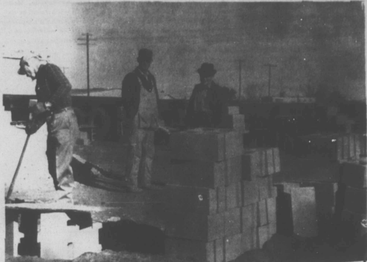
NEW BUSINESS FOR SUDAN-Work has begun on a new Shamrock Service Station to be located on East Hwy. 84. According to owner Arnold Reed, it will be a 30 x 40 concrete block building, with a grease rack to be located on the west side. Shown above is Shelby Morris, electrical contractor; S.P. Stockard, building contractor; Arnold Reed, owner; a brick-layer; and now shown is Luna Snow, plumbing contractor. (Staff Photo)
