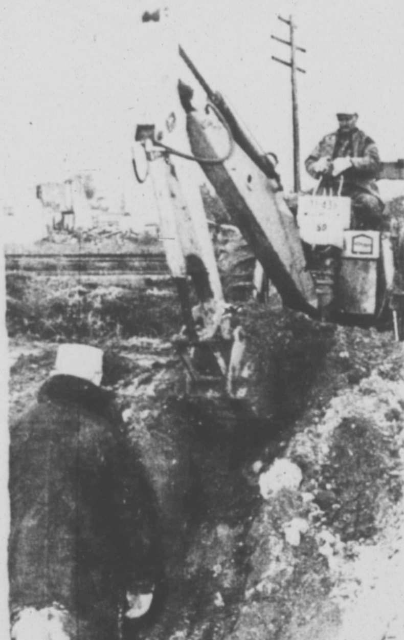
DIGGING FOR GOLD?—No, just the Sudan City employees digging for a main-line cutoff, when the Sudan main water line broke Tuesday night about 11 o'clock. The city workers stayed on the job all night, and service was restored to the Sudan area about 9:30 a. m. Wednesday morning. Fire Chief Pete Phillips is shown on the ditcher, and John Hendrix with his back to the camera.
