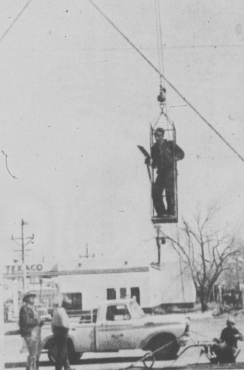
UP HE GOES --Shown above is a workman going up to the Sudan Water Tower, during the recent cleaning and repainting of the tower by the Pittsburgh Tank and Tower Company.
