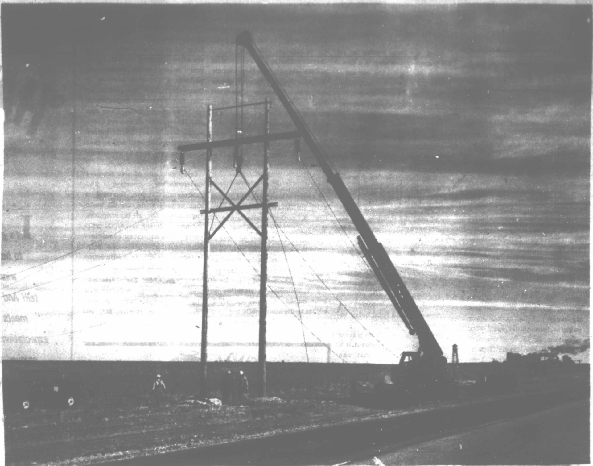
A PART OF SOUTHWESTERN PUBLIC SERVICE COMPANY'S $17,818,000 CONSTRUCTION PROGRAM FOR 1968 WILL BE ADDITIONS TO THE 4200 MILE TRANSMISSION LINE NETWORK SUCH AS THE LINES BEING INSTALLED BY THIS CONSTRUCTION CREW.
