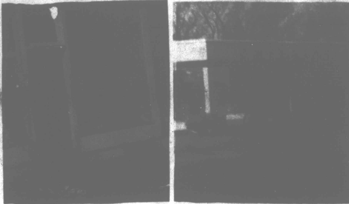
GLASS RAIN - It could have been raining glass by the looks of the drive Thursday morning at Nichols Phillips 66 Service Station. An explosion broke the plate glass in the front of the building and also did considerable other damage to the building.
