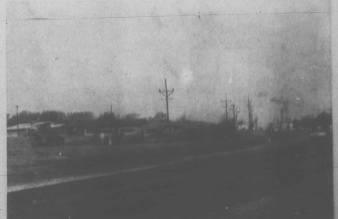
HIGHWAY 84 CONSTRUCTION got underway in a BIG WAY here this week as work crews began the removal of trees from the road right-of-way in preparation for the road bed of the divided highway. (Staff Photo)
