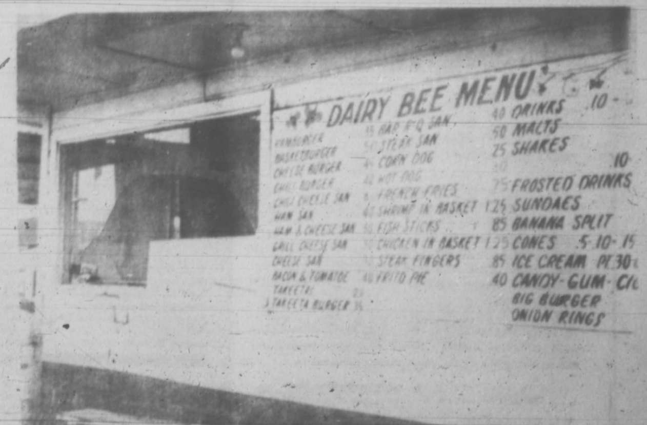
TRUCK DRIVE-IN - Shown above is the results of what happened to the Dairy Bee Drive-Inn when a truck wheel, which came off a moving truck ran into the side of the building. Ted Walker, owner reports the damage has been repaired and the drive-in is open for business.
