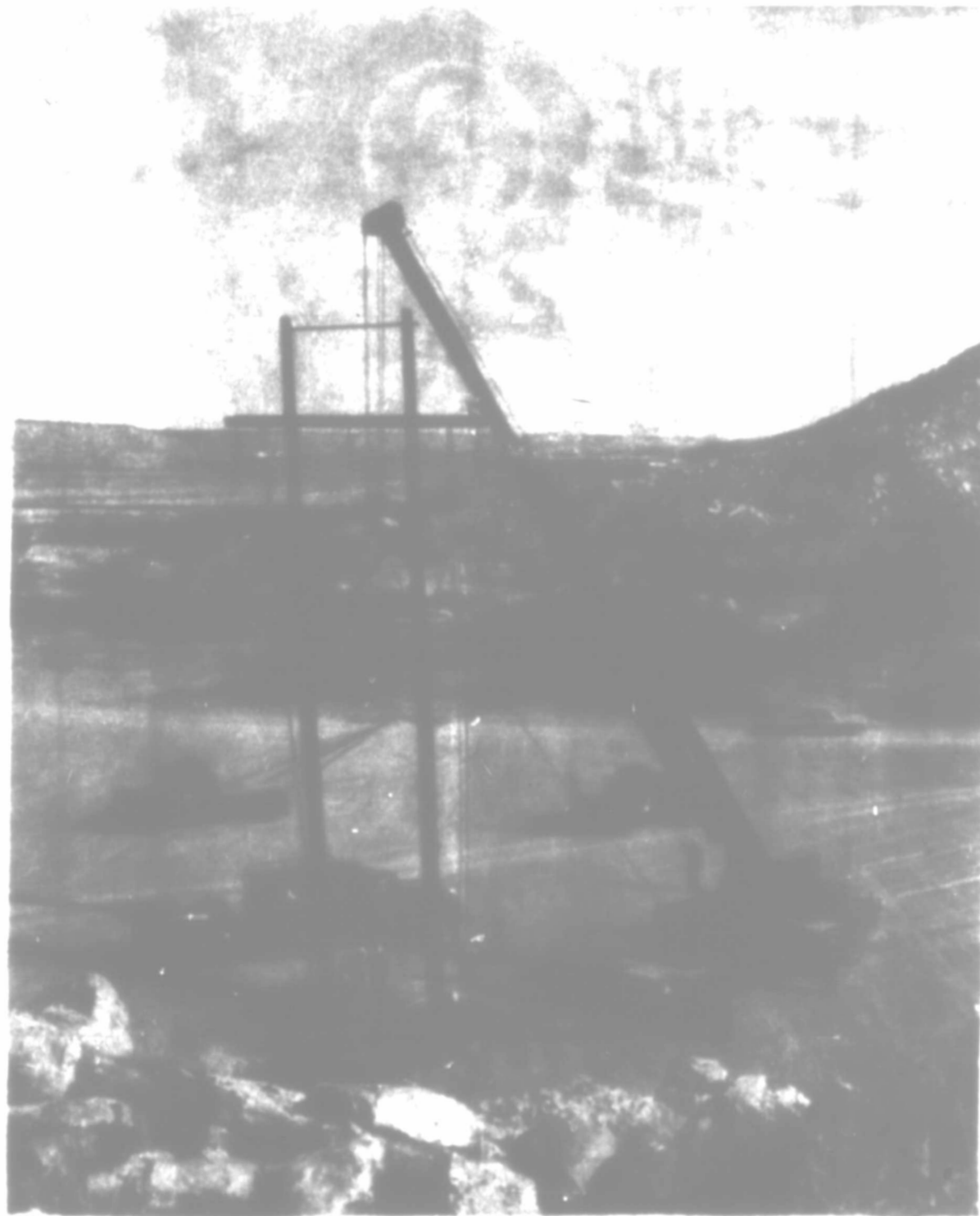
AN 80-ft. ELECTRIC TRANSMISSION line structure can be lifted and set into place in 8-1/2 minutes with Southwestern Public Service Company's new hydraulic crane. The unit, the second to go into service in the nation, was specifically designed for use in the electric utility industry. Southwestern Public Service has announced a 1966 construction program calling for the investment of $19,353,000 in new facilities, with a large part of the additional investment to be in transmission lines.
