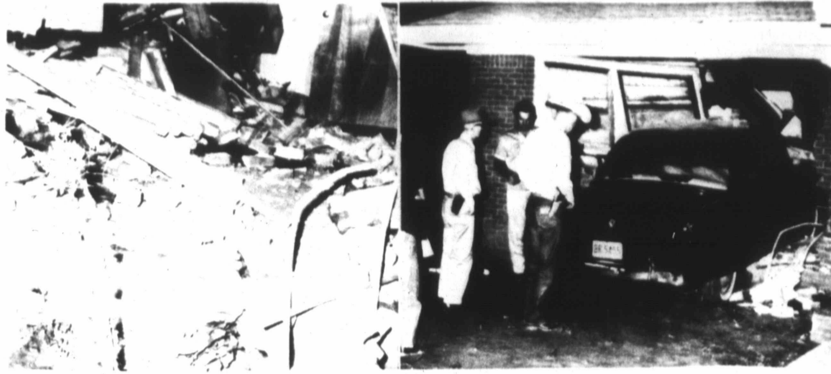
NO TORNADO — From the looks of the wreckage left in the bedroom at left, one might suspect a tornado had visited the home of Mr. and Mrs. John Withrow of Sudan. However, the mess was caused by the auto shown in the picture at right, which crashed into the house Friday night. Officers in the picture are Marshall Tom Hamilton, left, and Deputy Sheriff Homer McLaury. Driver of the car was Cecil Konkler, 23, who pleaded guilty of driving while intoxicated. (Staff Photos)
