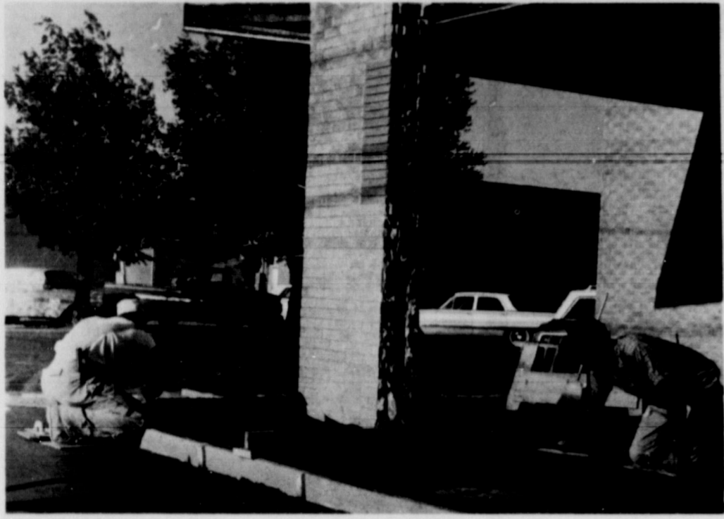
BANK ADDITION . . . A second drive-in window is under construction at Friona State Bank, and workmen are shown doing concrete work on the project this week.
