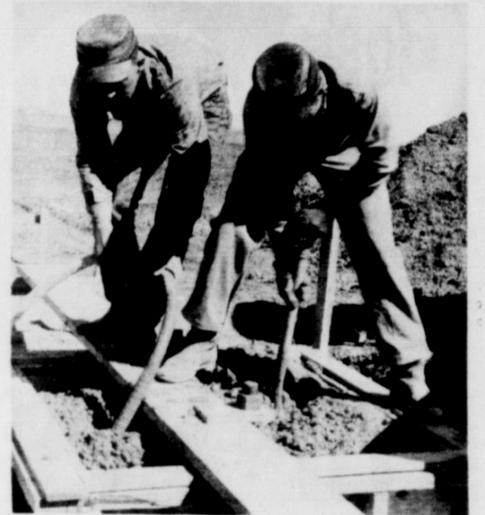
FINISHING TOUCHES . . . Workers are shown laying the final concrete for the foundation of Friona's new overhead water tower. Good weather allowed the operation to be completed in relatively short order.
