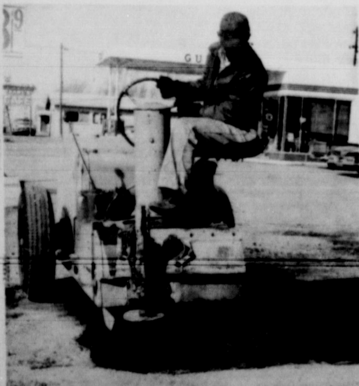
MAKING REPAIRS . . . City employees have been busy lately repairing holes in city pavements caused by the recent freezing weather. Here, Pete Hollis is busy making a repair on North Main.
