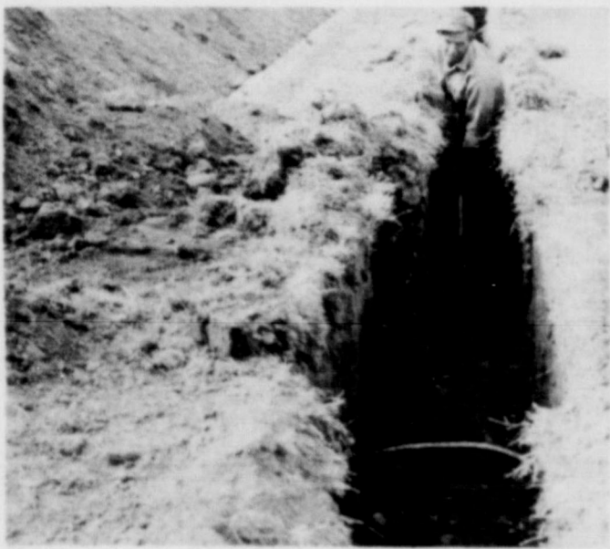
NEW PIPELINE . . . City employees are installing a new four-inch pipeline on Elm Street this week, in order to give residents a better water supply.
