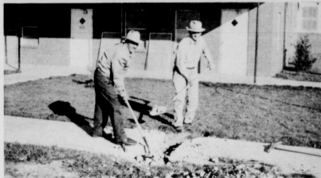
BREAK GROUND . . . El Roy Wilson (l), chairman of the building committee, along with H. A. Hyde, committee member, turn the first shovels of dirt for the new educational unit started this week by Calvary Baptist Church.
