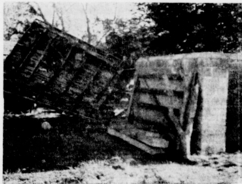
wellhouse roof up in trees
