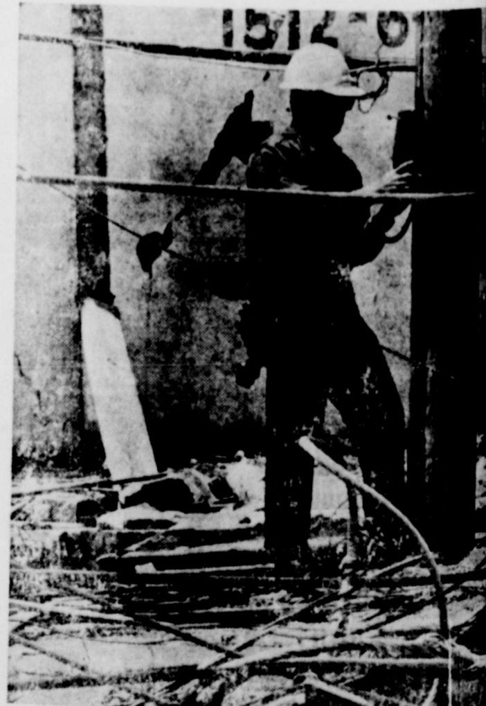
Telephone cable was cut up so badly it took installers like John Kins of Lubbock several hours to find working circuits and put emergency telephones into service throughout stricken area.
