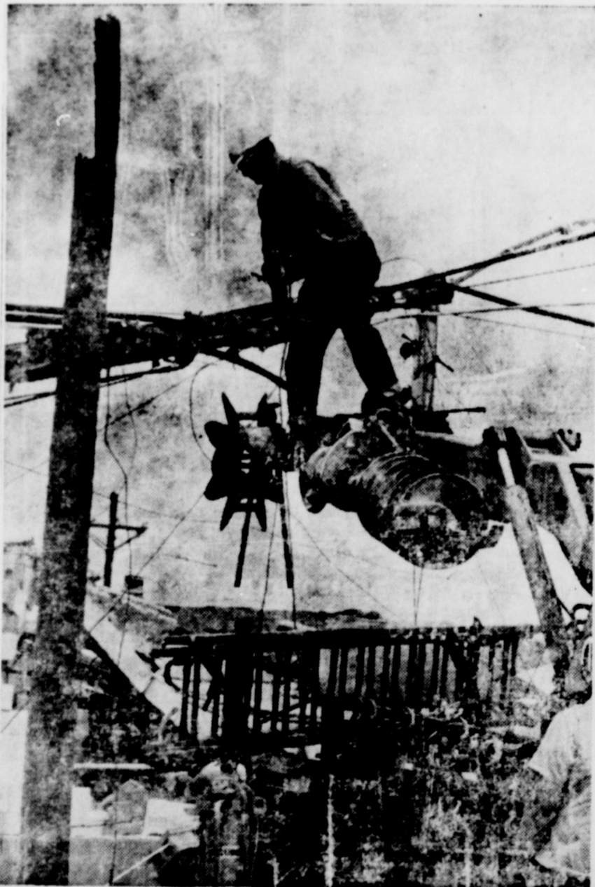
Cutting telephone cable loose from power lines after killer storm was major job for Dave Gammage, a lineman from Plainview.
