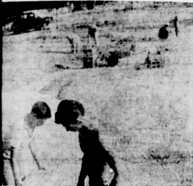
OFFER AND RONNIE SPRADLING apply the the cement sacks as workmen prepare a new for relocation of one of the school teacher- South of the S. E. Scott home.
