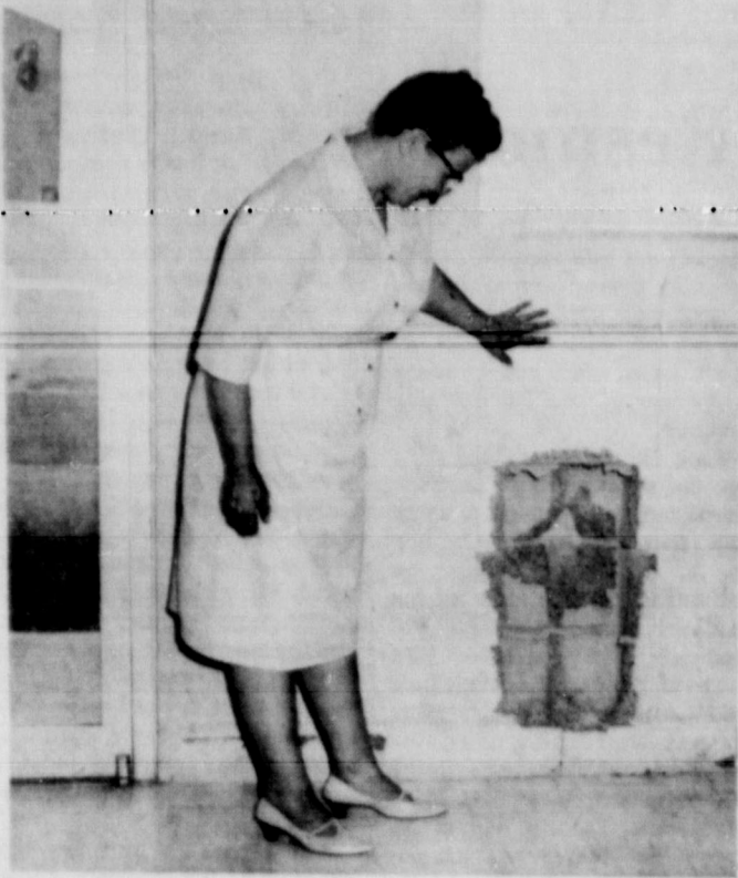
SURVEYS DAMAGE . . . Mrs. Pearl Johnson surveys damage to outside wall at Johnson's Food Market last week after a car driven by Mrs. Edward Montamayos crashed into the wall of the building.
