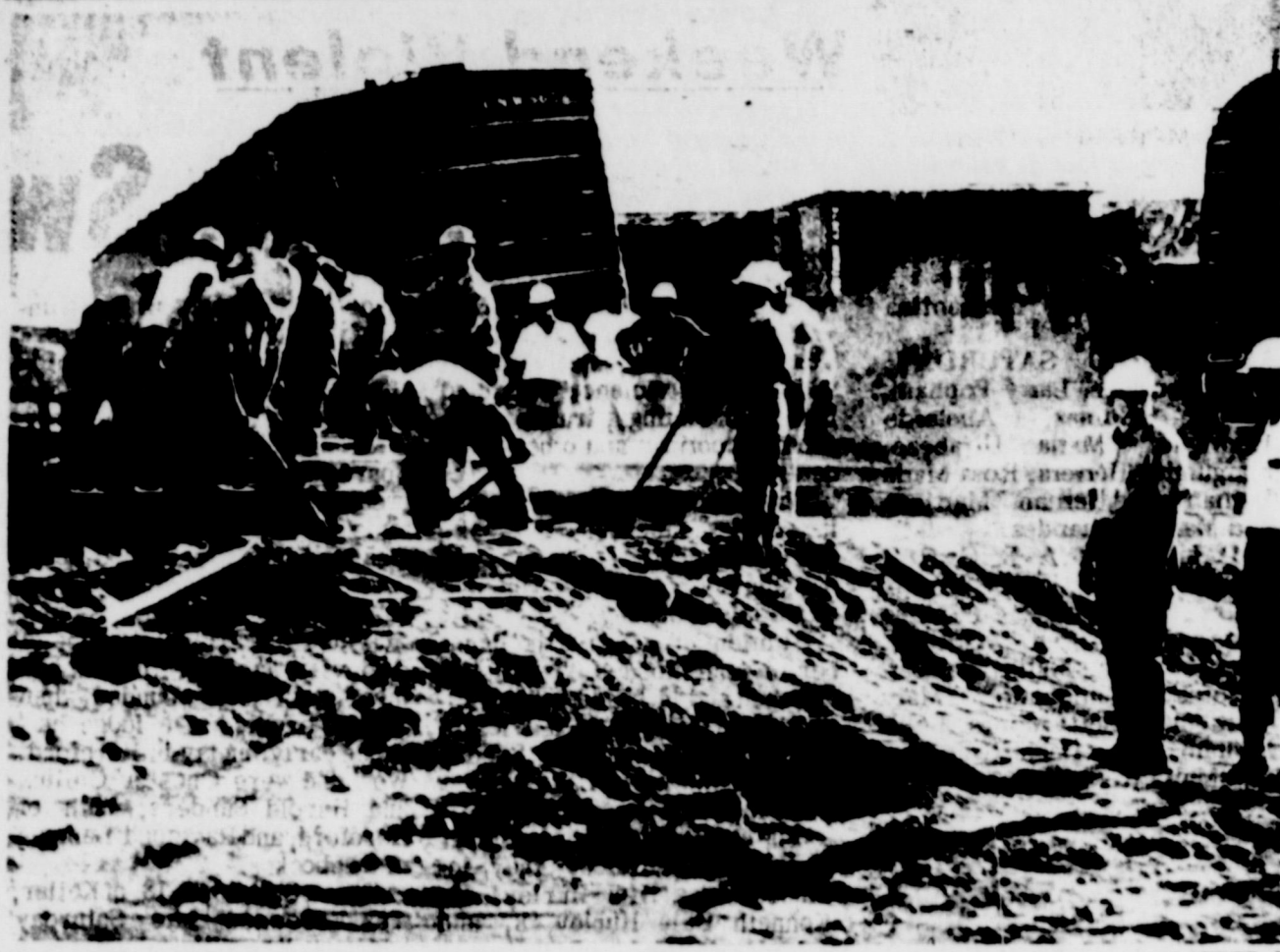
Southern Pacific relief crewmen rush completion of a "shoo fly" temporary track to carry traffic on the railroad's transcontinental mainline past 33 derailed cars blocking the railroad. An eastbound freight train derailed on the west side of Dryden at 8:15 a. m. Sunday. The line was re-opened for traffic at 7:40 p. m. Sunday. The picture was made on the north side of the wreckage looking toward the highway. (Del Rio News-Herald photo)
