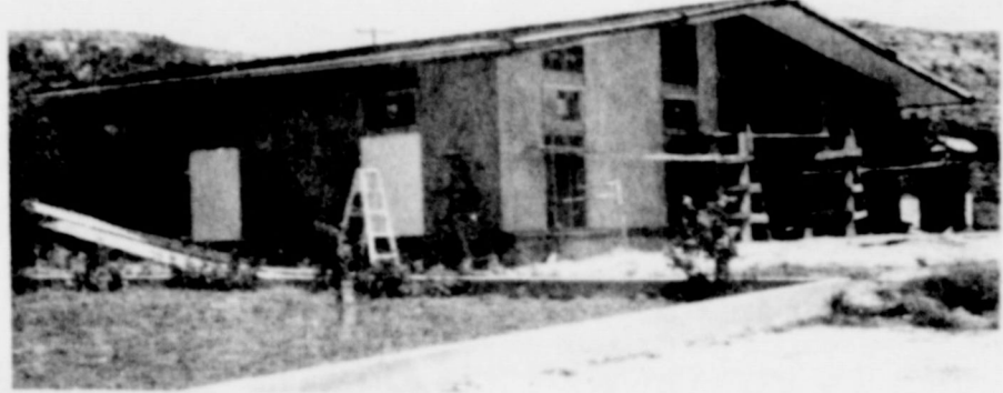
The Trans-Terrell Medical Center building is nearing the second stage of completion - the enclosing of the entire structure. The roof has been partially installed, paneling completely encloses the exterior, and some of the windows installed. The view above is from Persimmon St. and south of the building looking to the north. O. T. Sudduth is the contractor for the construction.
