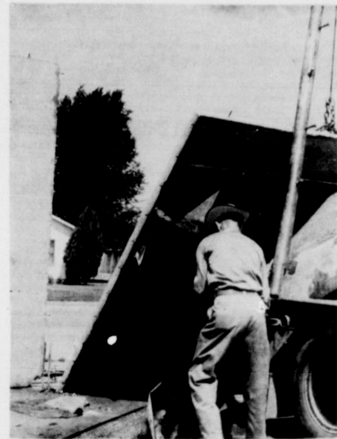
ANOTHER SECTION . . . A concrete section of wall is moved to its proper position, and will be set in place, anchored with concrete and steel.
