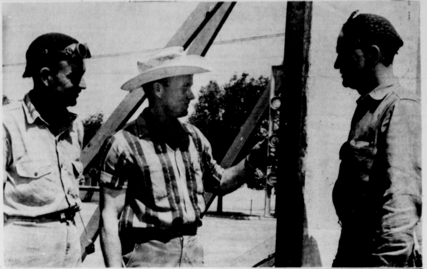
CHECKING ANGLES . . . Delton Lewellen, center, checks a portion of wall at building he is constructing of pre-fabricated concrete for Taylor and Sons. On the left is Ruben Taylor, and L. D. Taylor is at right.
