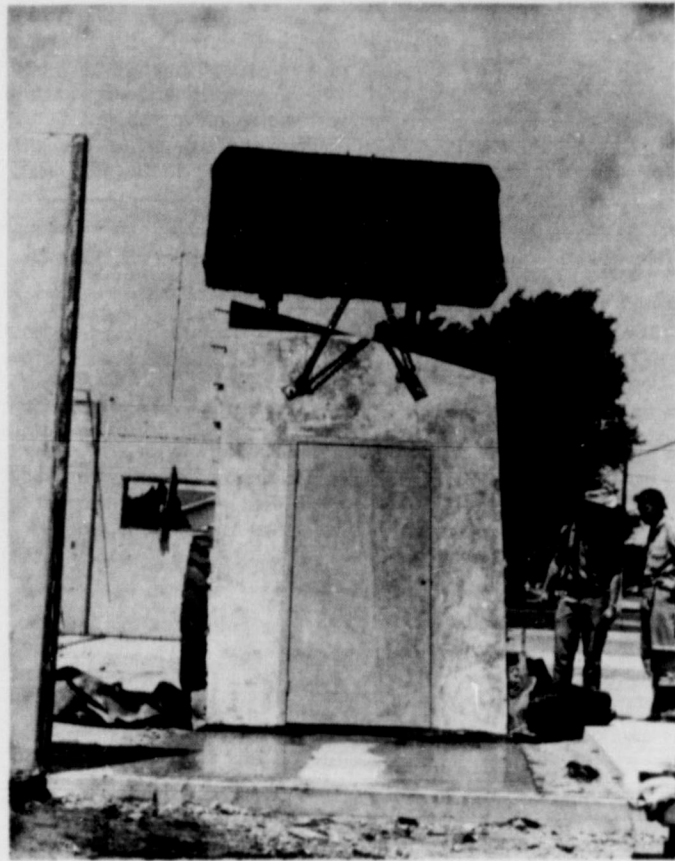
UP SHE GOES . . . A section of the wall at Taylor and Sons new blacksmith shop is hoisted in place and about to be anchored.
