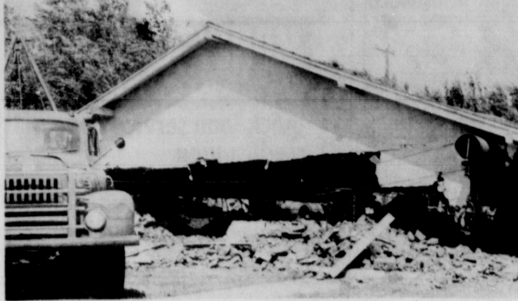
LANDMARK COMES DOWN . . . The old Methodist Church building, one of the city's landmarks, was torn down this week to get ready for a new educational building which the church will build. The old structure was erected in 1924.
