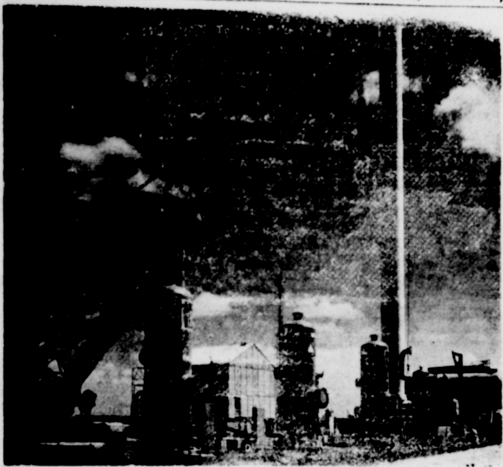
NEARS COMPLETION — El Paso Natural's treating plant in Terrell County is expected to be on stream before the end of the year. The tall stack, seen at the right, will be used to disperse carbon dioxide, removed from field gas, high in the atmosphere. Field gas, taken from the Ellenburger formation of the Brown-Bassett multiphase field, has been tested at slightly more than half carbon dioxide.
