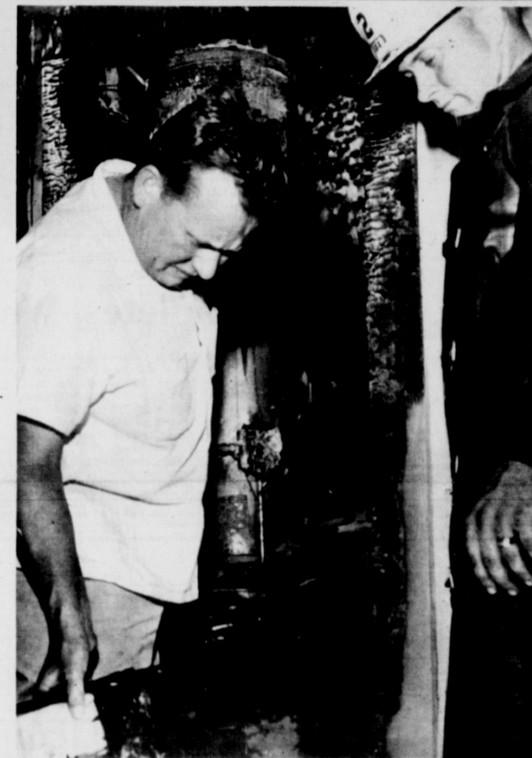
FIRE SOURCE . . . Friona Fire Chief Ralph Shirley and Glen Reeve, Jr. examine water heater closet, which was the source of the fire at the Cecil Floyd residence last Friday.
