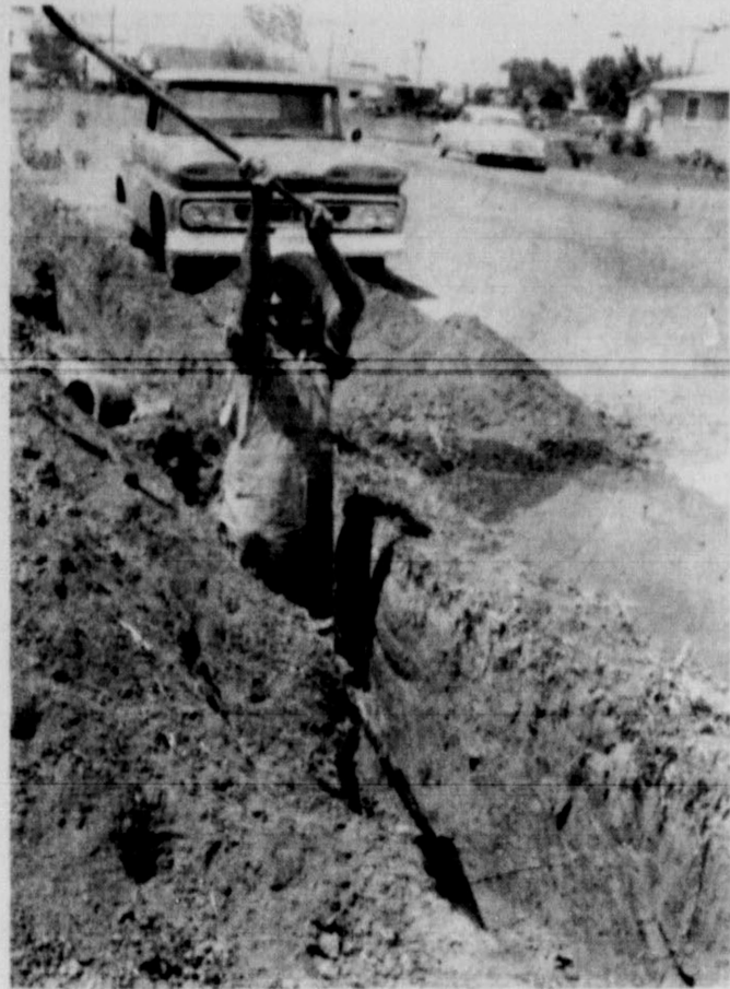
COOL PLACE TO SPEND SUMMER--Howard Love shows how to dig a ditch as city workmen move a fire hydrant at the location of the new White Supermarket in Friona. Really Love didn't dig all this ditch with a shovel, but by the size of sweat drops he looked as if he had.
