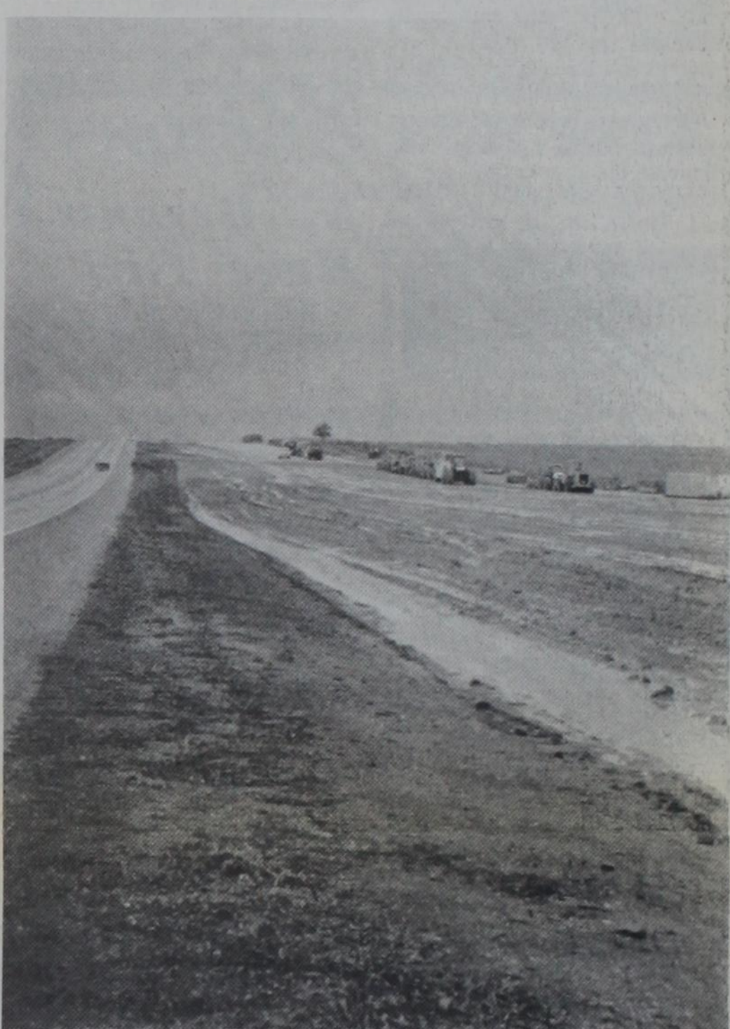
RAINED OUT.... Construction of U.S. Highway 60 near Caprock Industries came to a halt Tuesday morning, July 20, as rain made conditions sloppy. Nearly one-half inch of rain fell from 5:30 a.m. until around 11 a.m.
