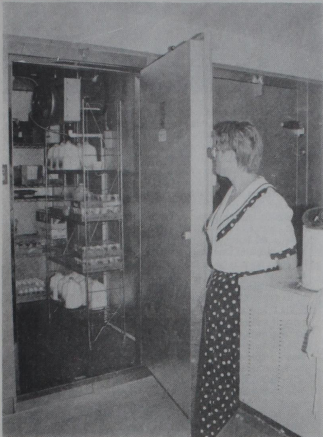
BEFORE AND AFTER.... Jo Blackwell, Prairie Acres, holds the door open to the new walk-in freezer and refrigerator. The walk-in is one of the many projects the nursing home recently finished.
