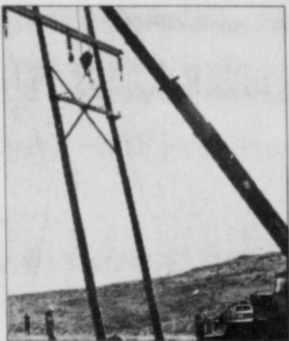
"We're putting in a new 115,000 volt line . . . gives us another feed to back up our dependability . . ."
