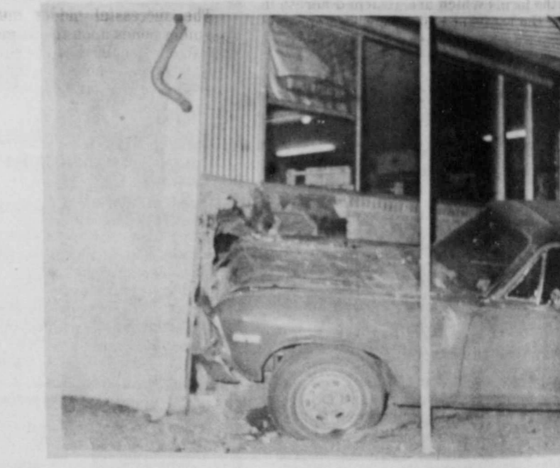
THIS CAR DRIVEN BY Floydada High School sophomore Kristi Love crashed at Bishop-Ramsey Pharmacy Saturday night. Kristi just missed the driver's door. The building was insured and police officials said no charges had against Kristi at press time.
